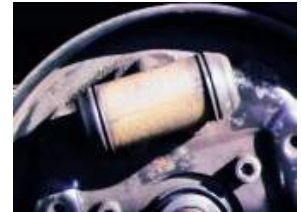
Check carefully for any brake fluid leak (under the dust boot)
